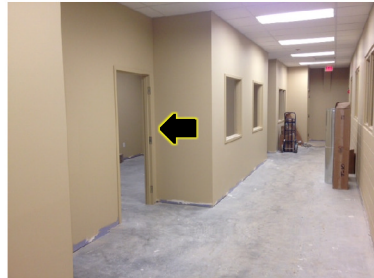
This is the entrance to the room to be named for the club.
